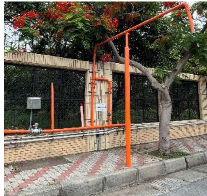
Reclaimed Water Collection Point
