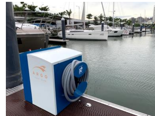
wastewater pumping equipment
